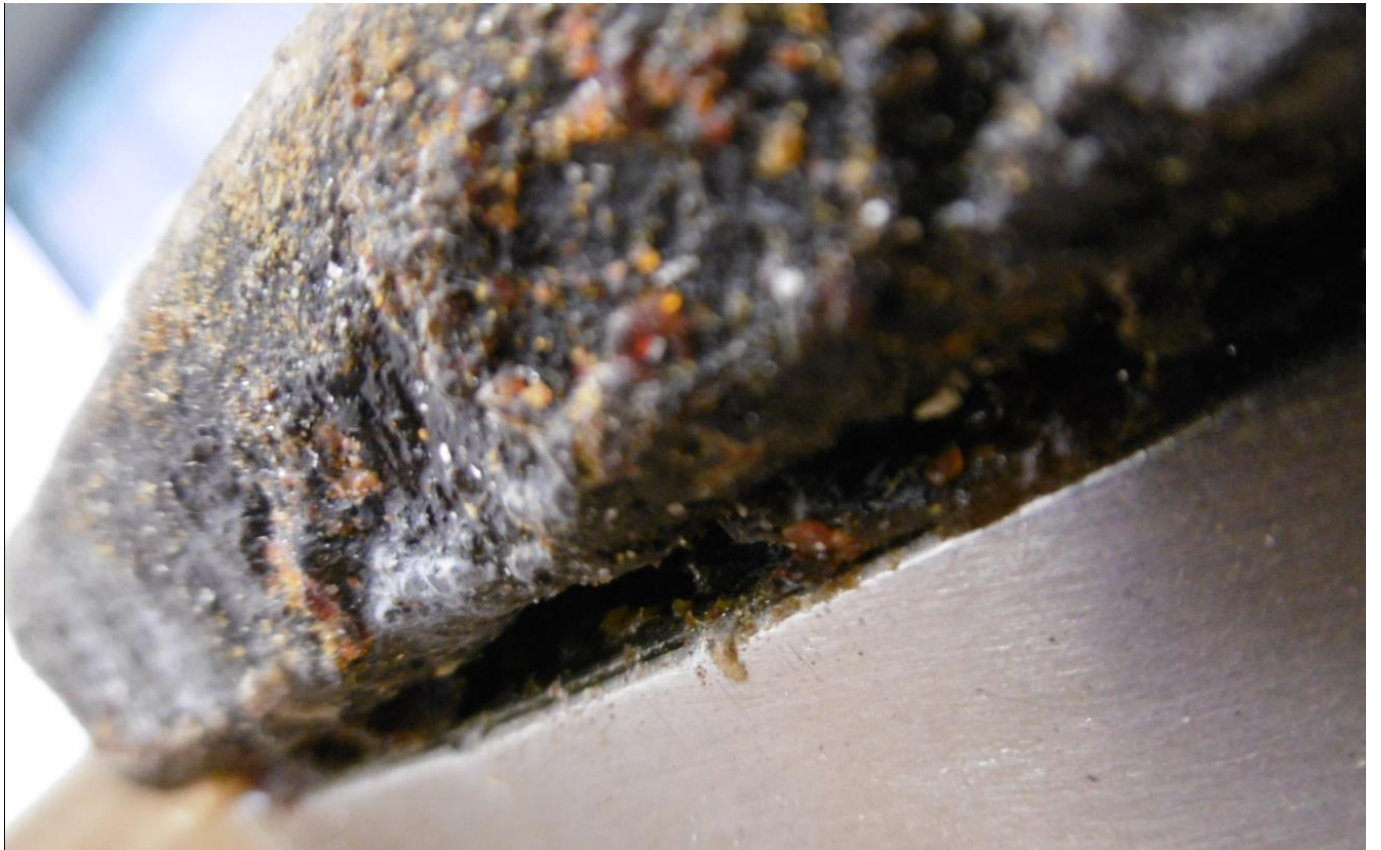
SURFACE OF HEATING PLATE– visualization of not cleaned & maintenance surface [out of warranty]
